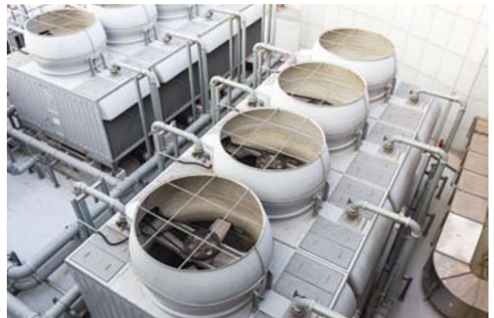
Cooling towers, an application where HTH Scientific® Chips & Granular can be used.
